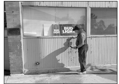
Tim Fugman worked on scraping and removing grime with a pressure washer.
